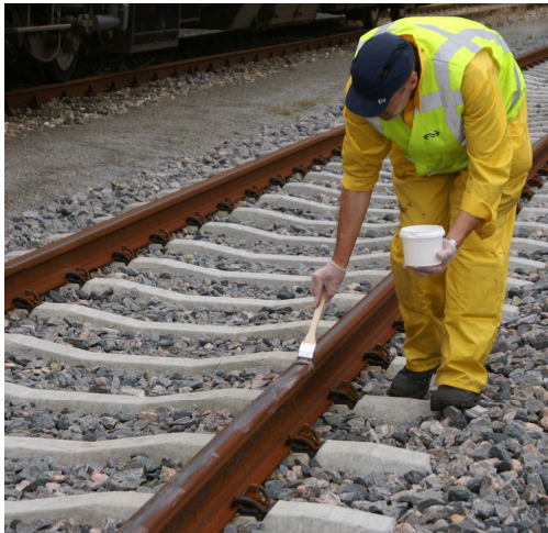
Figure 6.3 Applying grease to the rails in order to make the track slippery.
