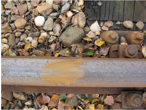
Figure 6.1 Rust on the rail
